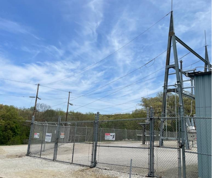
CIPCO Winterset Junction Substation near Winterset
