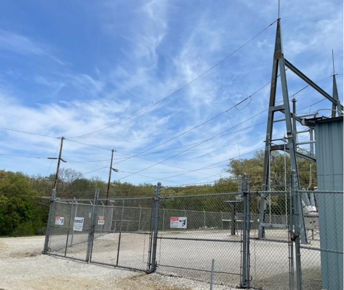
CIPCO Winterset Junction Substation near Winterset
