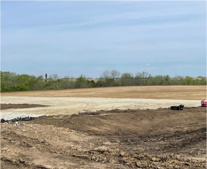
Future Site of new Alliant Energy and ITC Midwest Yaholi Substation near Osceola
