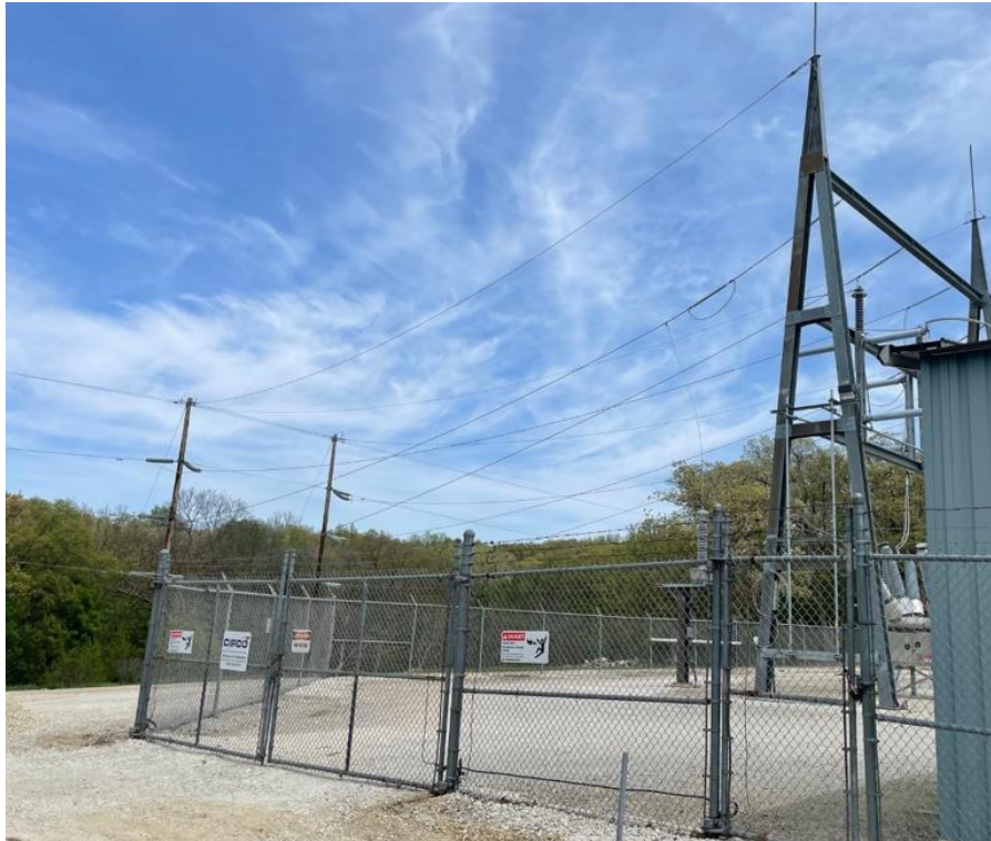
CIPCO Winterset Junction Substation near Winterset.
