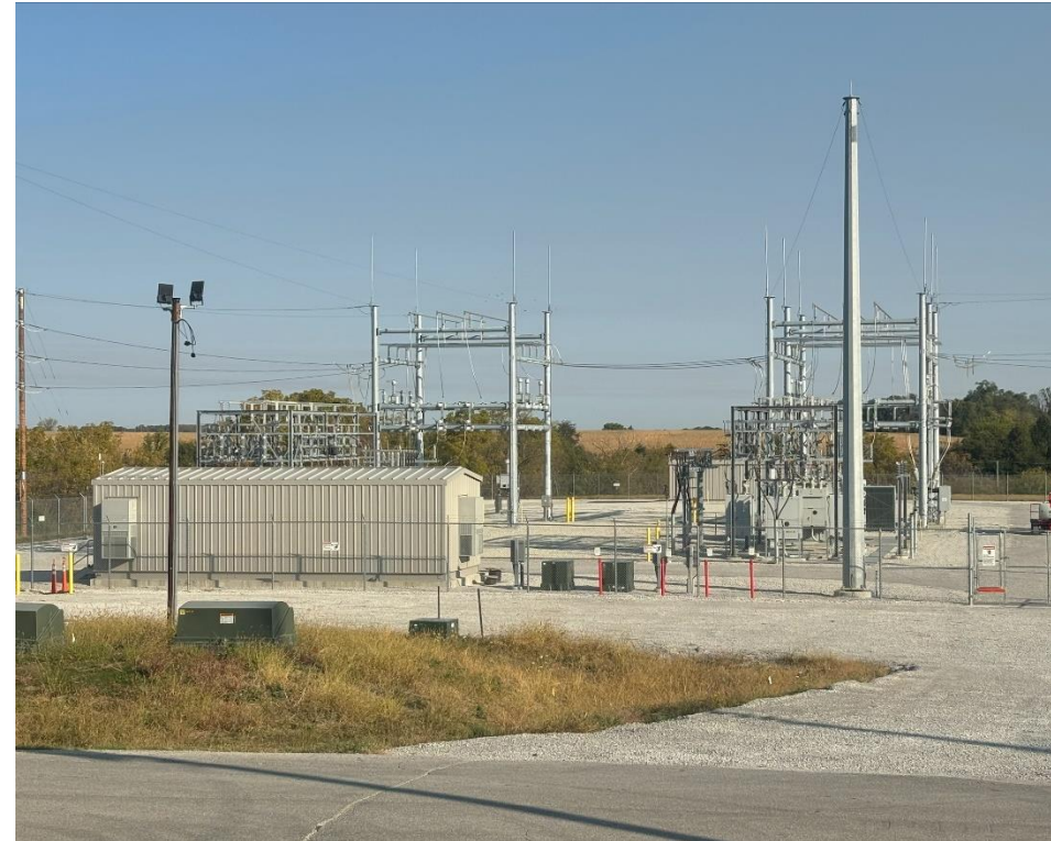
Site of the Alliant Energy and ITC Midwest Yaholi Substation in Osceola.
