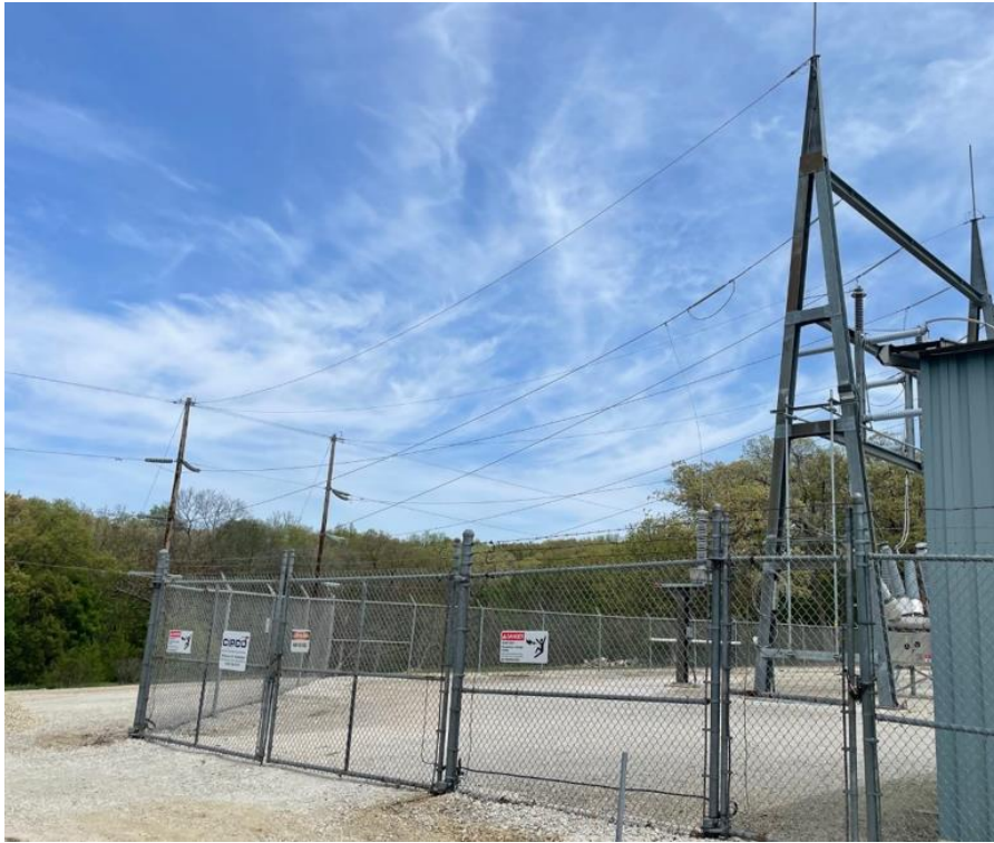
CIPCO Winterset Junction Substation near Winterset.
