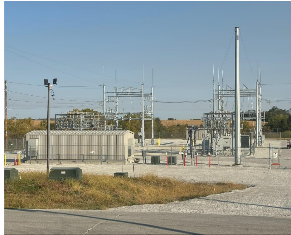
Site of Alliant Energy and ITC Midwest Yaholi Substation in Osceola.
